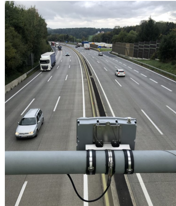
C-ITS units as part of ASFINAG 's infrastructure
